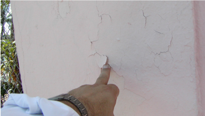
Photograph 1: Impermeable Paint - If the paint on the stucco is too impermeable it bubbles, blisters and peels. The paint on the stucco needs to be greater than 10 perms "wet cup" or it will bubble, blister and peel.
